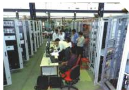
Customer inspection during integrated FAT (Factory Acceptance Test) at Pallavaram unit for Control relay panels
