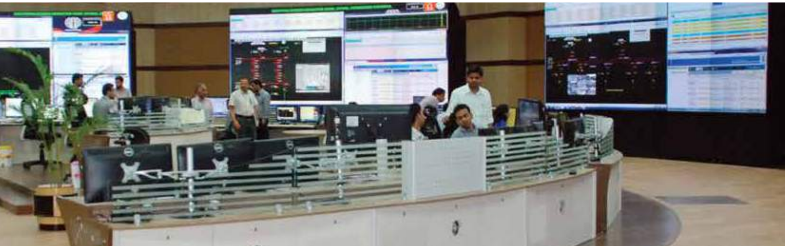
National Transmission Asset Management Centre at Manesar successfully commissioned
