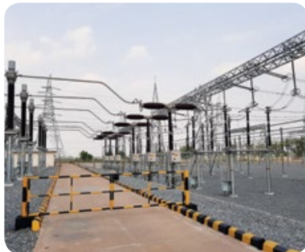
▲ 400 kV Air Insulated Substation for Odisha Power Transmission Corporation Limited (OPTCL) at Lapanga, Odisha
