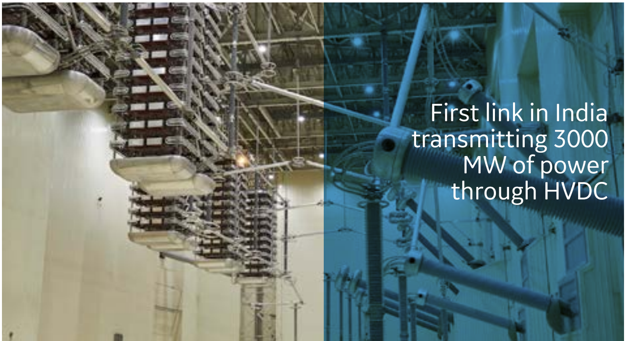
Valve Hall 765 kV HVDC at Kurukshetra
