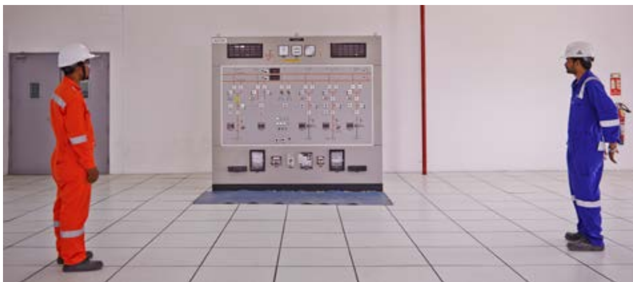
Grid Automation Unit - Pallavaram
