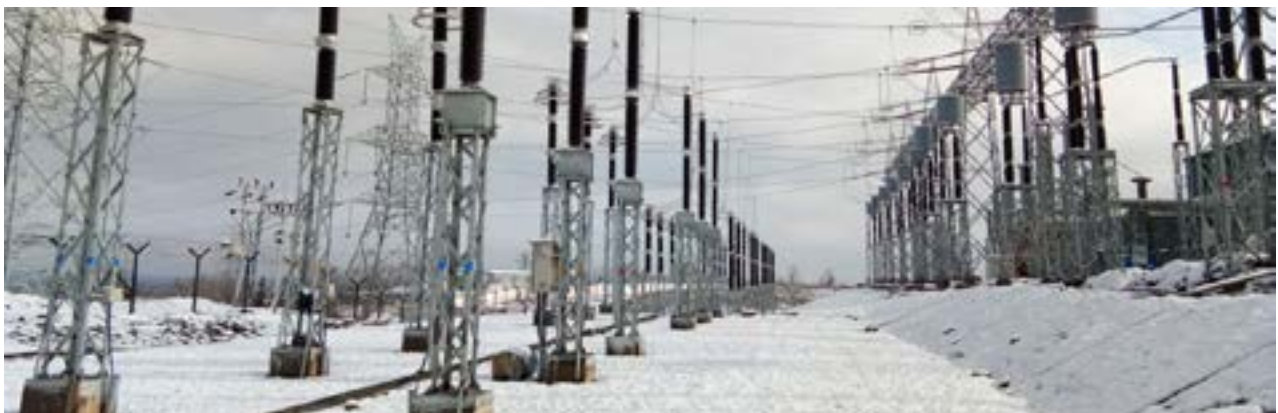
400/200 kV Gas Insulated Substation situated at an altitude of 2024 mts (6640 ft) in the Amargarh village of Kashmir
