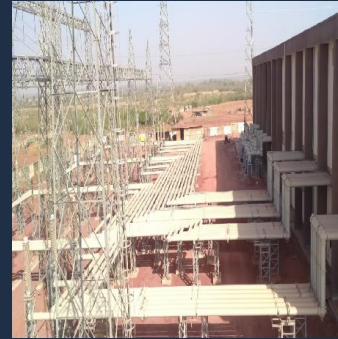
GETCO Shapar, Gujarat Commissioning of 400 kv 12 bays and 220kv 15 GIS bays
