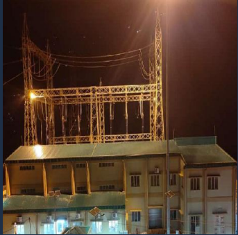
HPPTCL, Hatkoti, HP – Commissioning of 220 kv 7 GIS bays
