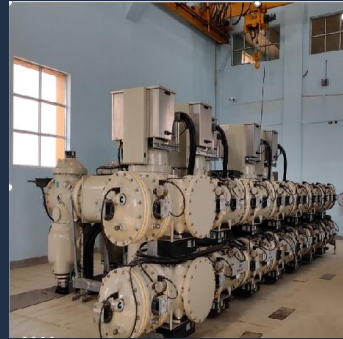
WBSETCL Manbazar Full Commissioning of 132kv 6 GIS bays , 33kv 15 GIS bays and 2x31.5MVA transformer Substation
