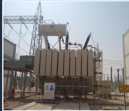
5x220kV AIS Bays, 3x33kV Switchboards with 3x125 MVA Transformers for 300MW Solar Plant evacuation commissioned for Surya Urja at Bikaner
