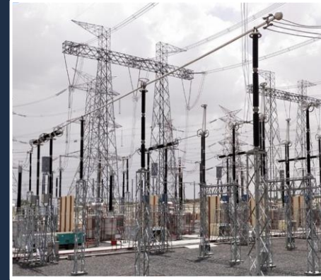
2x765kV AIS Extension Bays with 7x 80MVAR Line Reactors charged successfully for Adani BKTL at Bikaner
