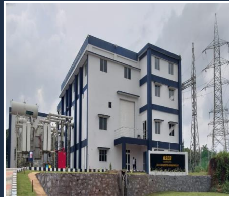
220kV GIS along with GIB & 2x100 MVA ICT commissioned at KSEB Kunnamangalam
