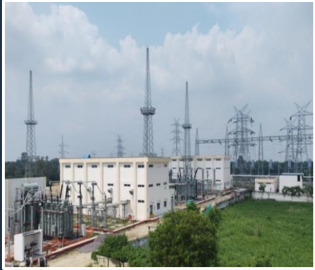
8x400kV bays, 4x220kV, 5x132kV GIS Bays, 2x500 MVA ICTs along with 1x63 MVAR Bus Reactor commissioned at UPPTCL Hardoi Road
