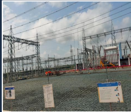
12x400kV, 8x220kV AIS bays with 2x500 MVA ICTs & 2 x 125MVAR reactors commissioned for NKTL Adani at Dhanbad
