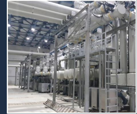
1 Bay along with line successfully charged for Doosan at Obra
