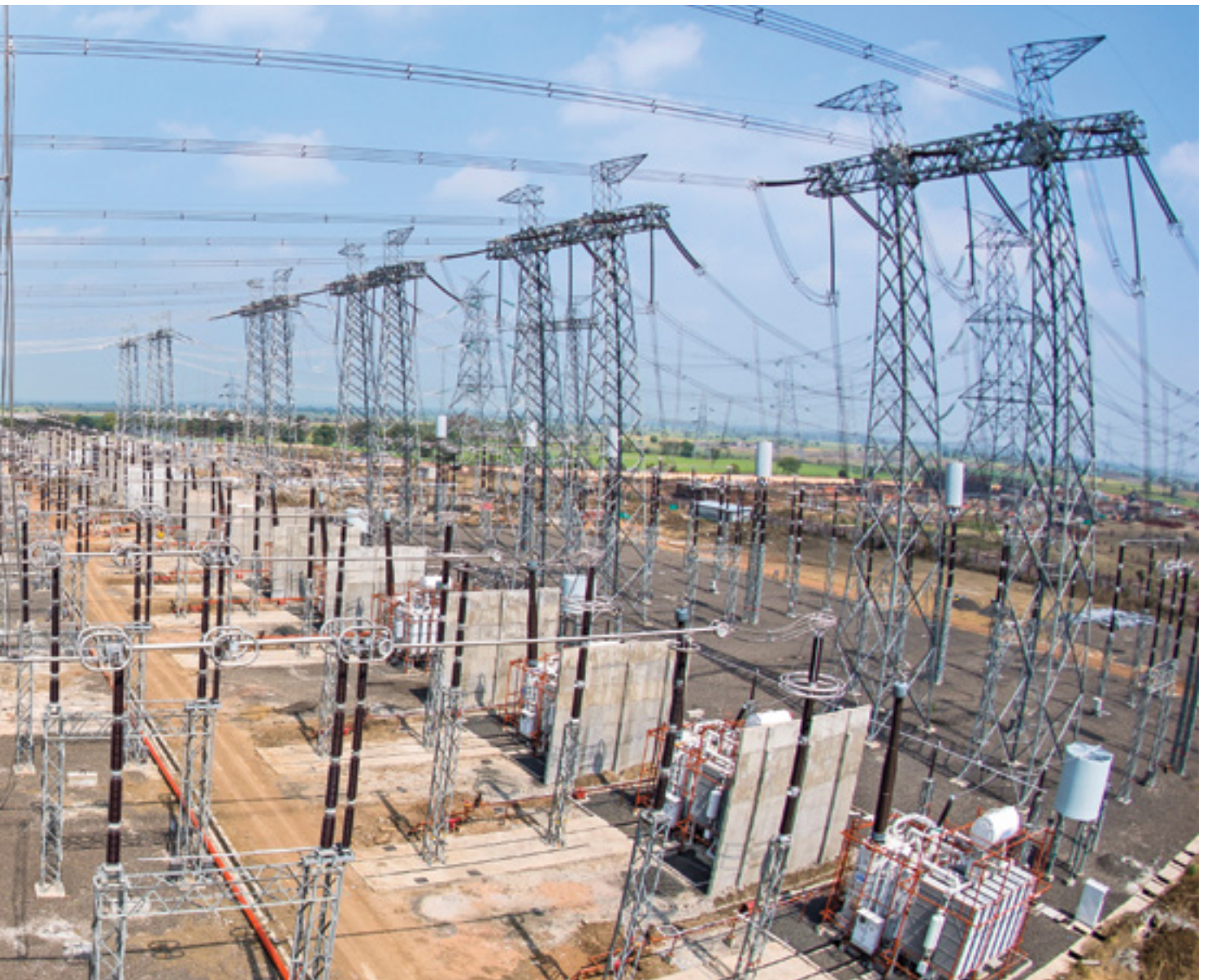
▲ Air Insulated substation at Bina
