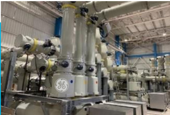
Commissioned 220/132/33 kV AIS for BSPTCL at Supaul
