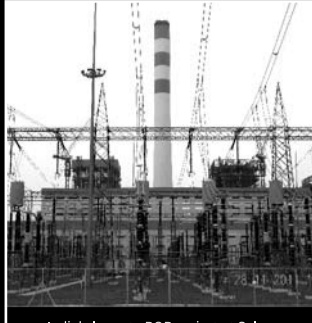
India's largest eBOP project at Salaya
