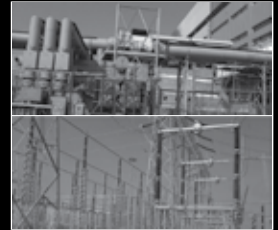
eBoP & 400 kV switchyard for 300 MW Warora Power Plant
