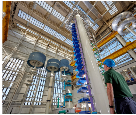
High voltage test lab at the power transformer factory in Stafford, United Kingdom
