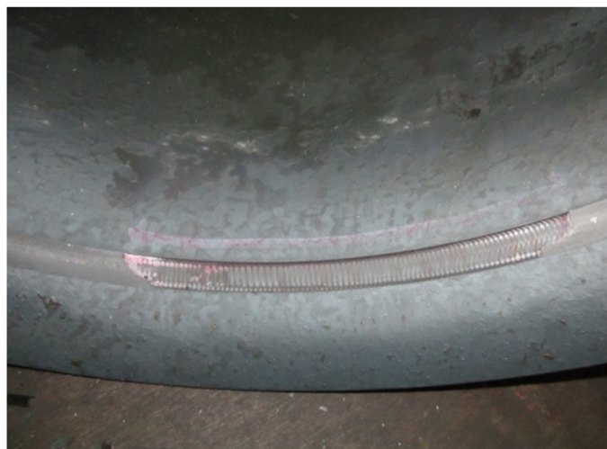
Cracking on the contact surface of a valve seat
